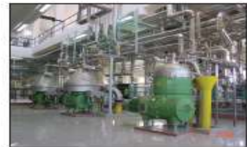
A piping network in an industrial facility.
